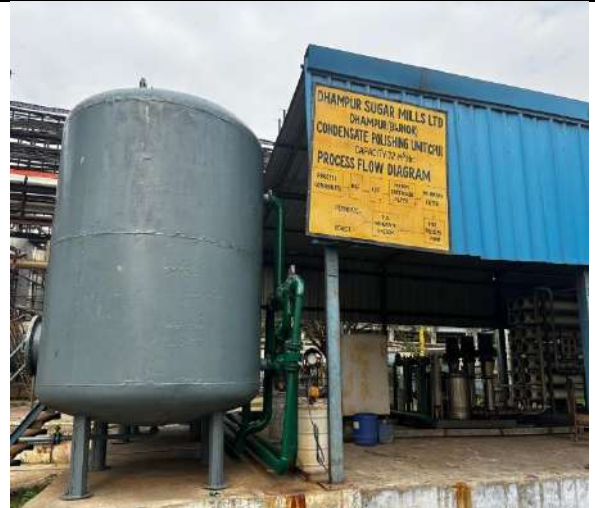
Fig 8: Condensate Polishing Unit
