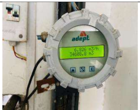
Pic: 8 Flow meter at the inlet of STP
