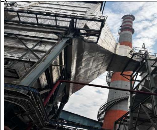
Fig 9: Common stack for both boilers
