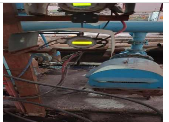
Pic: 6 Flow meter at the outlet of ETP
