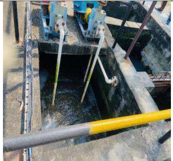
Pic: 10 STP inlet
