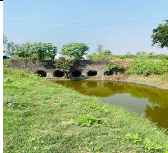
Pic 16 : Rain water accumulated in River SOT
