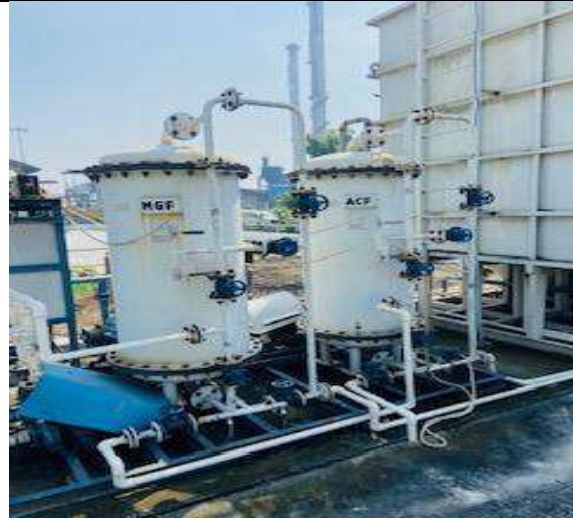
Pic: 11 MGF and ACF units of STP
