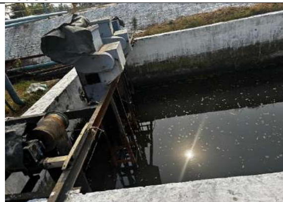
Pic 4 : Oil and Grease tank
