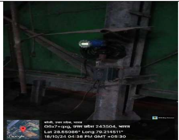
Pic 2: Flow meter at the mill boiling house
