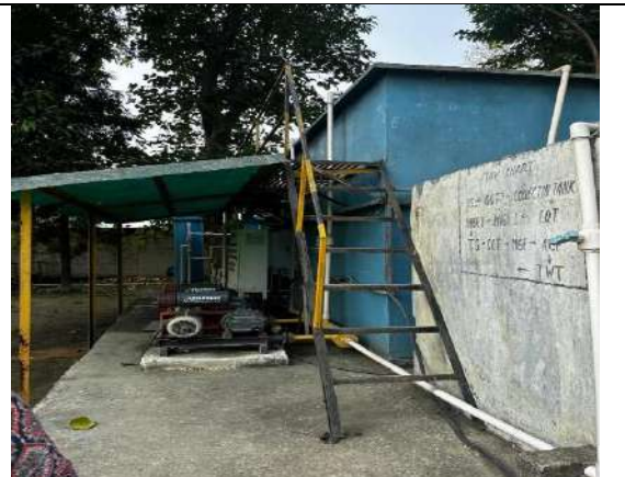
Pic 6: Sewage Treatment Plant
