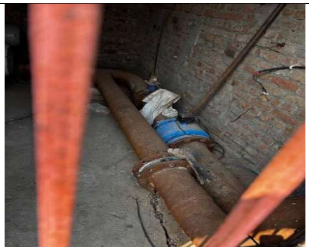
Fig 4: Pipeline from lagoon for irrigation
