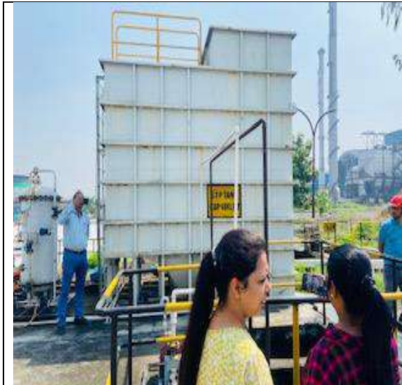
Pic: 9 Sewage Treatment plant
